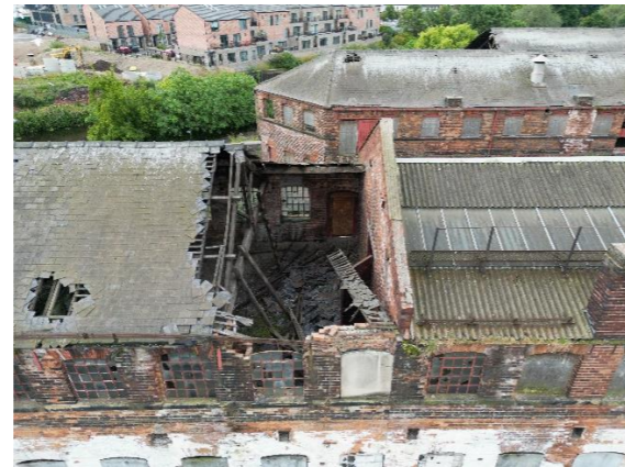
Figure 27: At the east the roof has collapsed exposing the timber trusses and floors to the elements. The building fabric is substantially damaged and decayed in this location.
