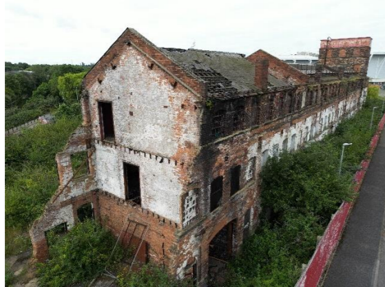
Figure 26: The east end has substantially deteriorated following the demise of the connecting wing. The cross wall and its openings are open to the elements, permitting water into the building.
