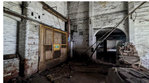
Figure 29: At the ground floor several openings have been boarded up or infilled with brickwork.
