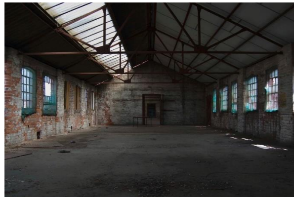
Figure 28: The third floor to the central bays shows the steel trusses and rooflight.
